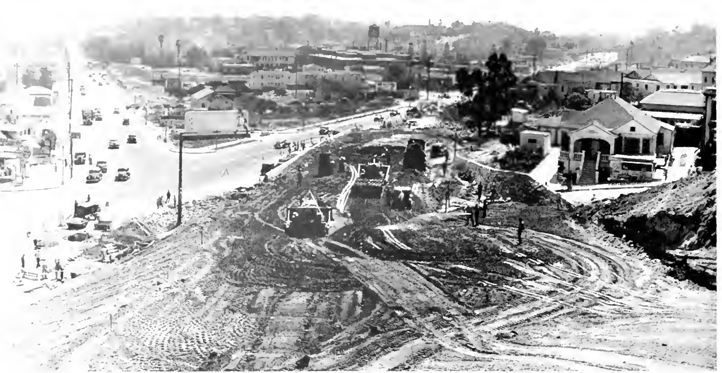
Extensive grading work and site of two overhead grade separation structures at intersection of Castelar and Figueroa Streets
